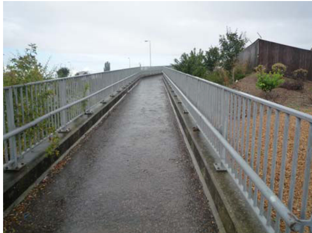
Poor colour contrasting handrails
