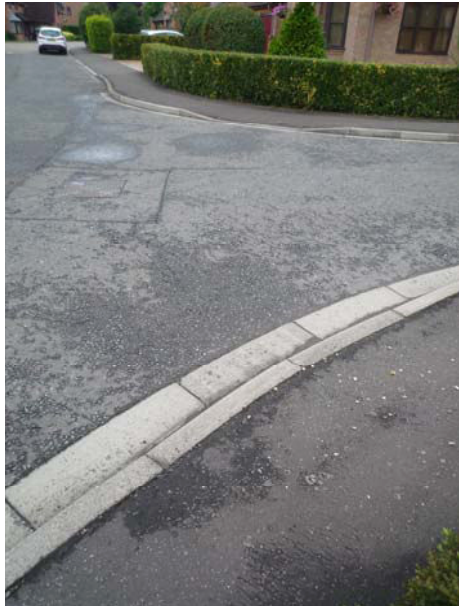
Dropped kerb location with no tactile warning
