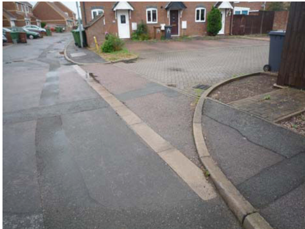
Dropped kerb but lacking in tactile paving
