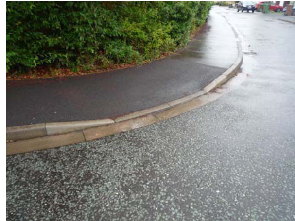
Dropped kerb with no blister warning
