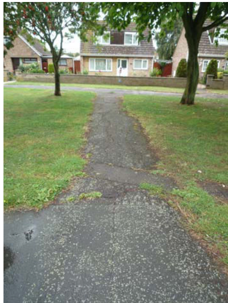
Path showing the early sign of breaking up
